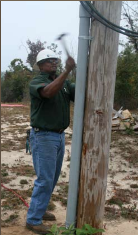
Clarke-Washington EMC lineman, David Bryant attaches a conduit bracket to a power pole.
