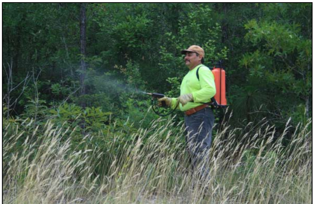
Crews sprayed about 900 miles of rights-of-way this summer. Here vegetation is being sprayed with herbicide to keep these areas clear of brush.
